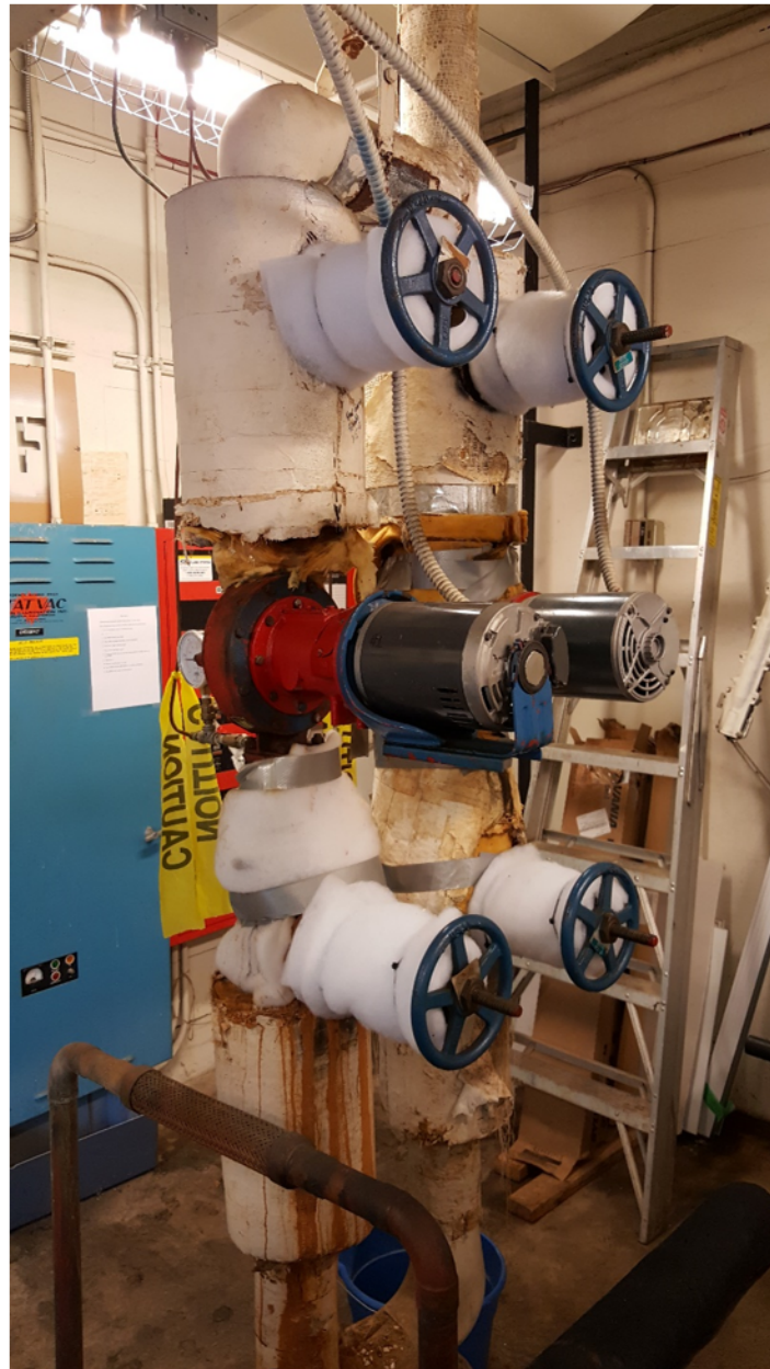
Photograph #2 – Chilled Water Piping and In-line Pumps
