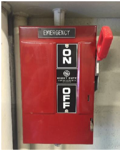
Photograph #17 – Disconnect to Serve Fire Alarm System
