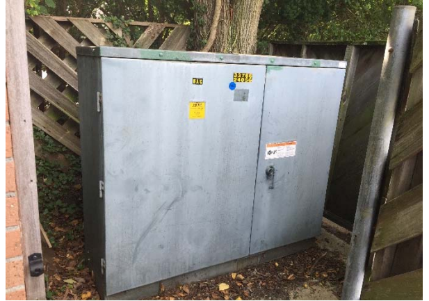
Photograph #14 – Delmarva Power Pad-Mounted Transformer
