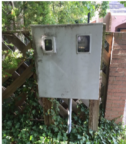
Photograph #15 – Metering Cabinet Containing Two Meters
