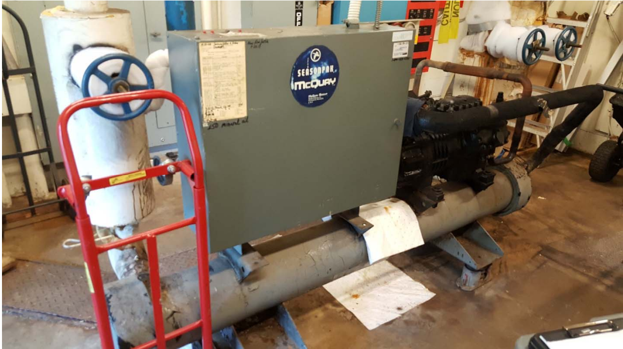
Photograph #1 – Air Cooled Chiller
