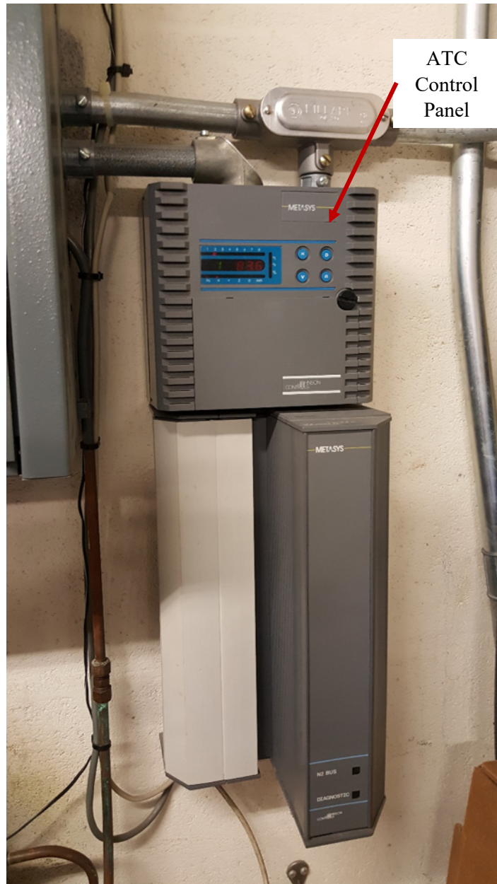
Photograph #12 – ATC Control Panel
