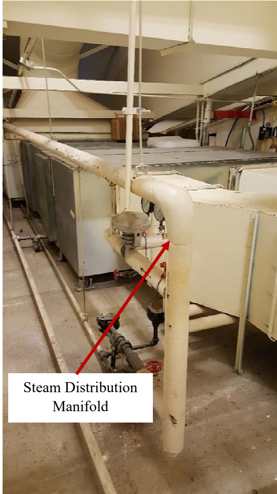
Photograph #9 – Steam Humidifier
