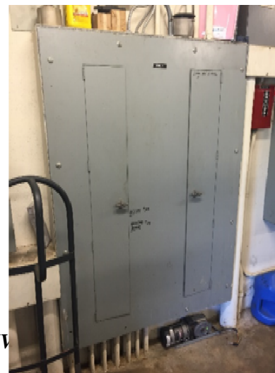
Photograph #20 – Panelboard “B”
