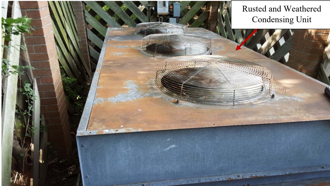
Photograph #3 – Existing Condensing Unit
