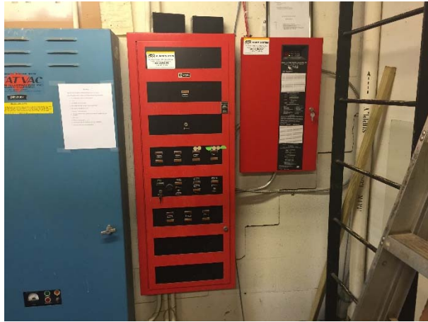
Photograph #18 – Fire Alarm System and Abandoned Emergency Lighting System
