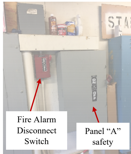
Photograph #16 – Panel “A” Fire Alarm and Disconnect Switch
