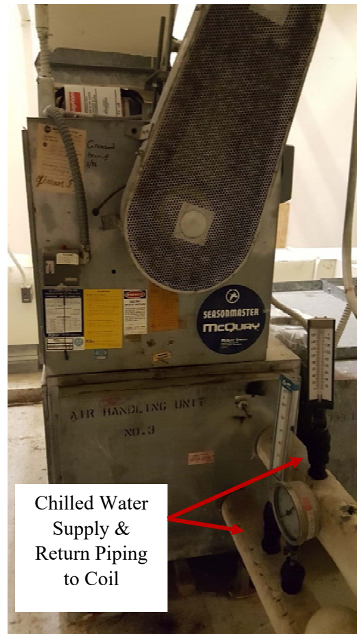
Photograph #8 – Air Handling Unit #3
