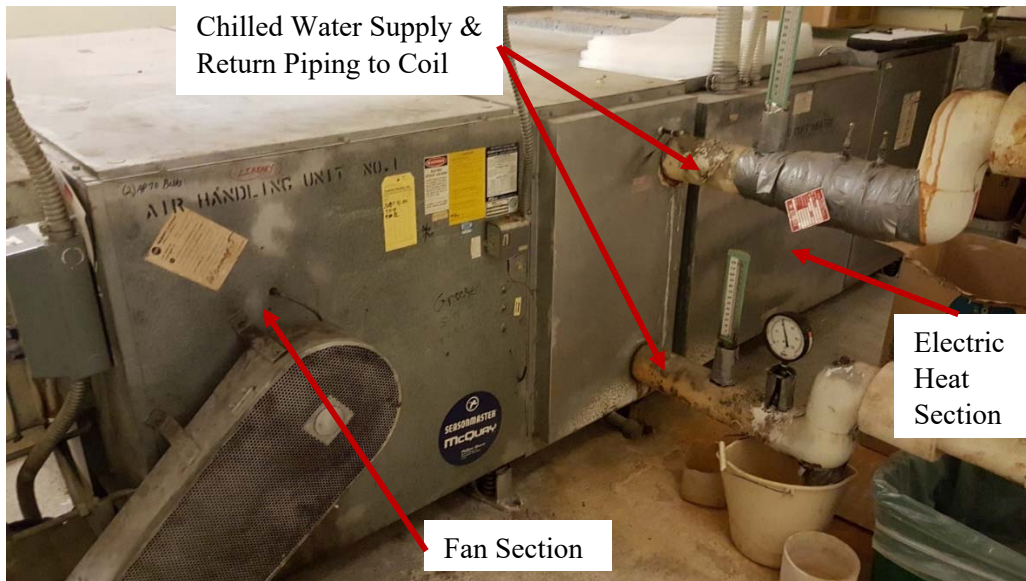
Photograph #4 – Air Handling Unit #1
