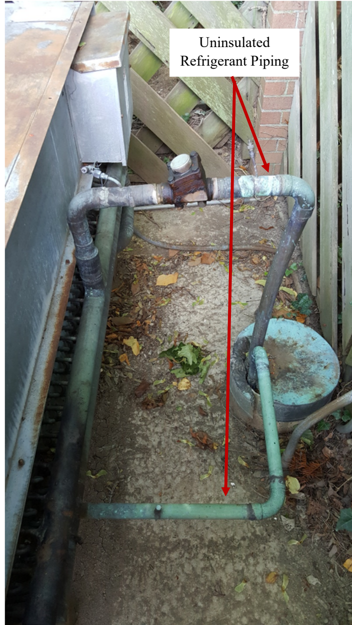
Photograph #4 – Refrigerant Piping from Condensing Unit
